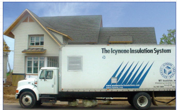
Icynene® insulation and air barrier system was installed because its air-sealing property helped improve indoor air quality and comfort for the Knight family, which includes a daughter with asthma.
