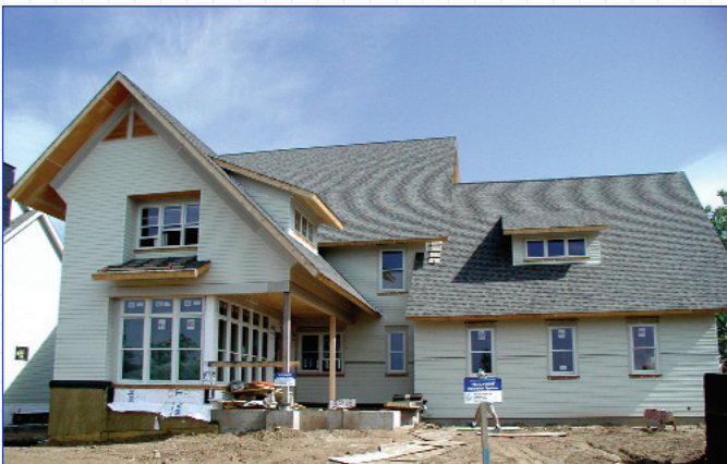
While working with the ALA, Chuck Knight was inspired to build his own 5,200 sq. ft. Health House in Woodbury, Minnesota.
